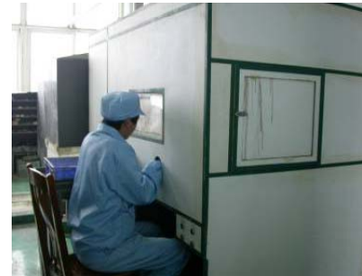
Pre-plated Treatment Equipment
